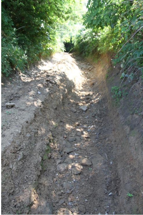
Part of Back Lane is now a trench
